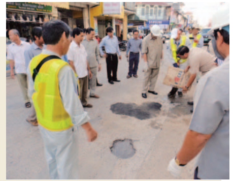
Using the Asphalt Repairing Material (EXCEL) to repair damaged road areas. (Photo: IKEE Group)
